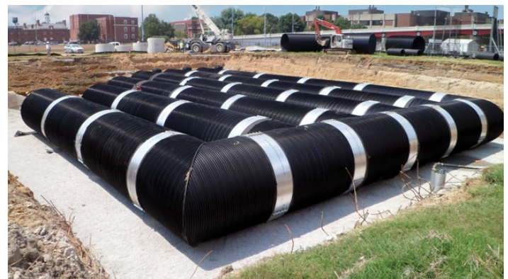
BELOW GROUND RETENTION BASIN
